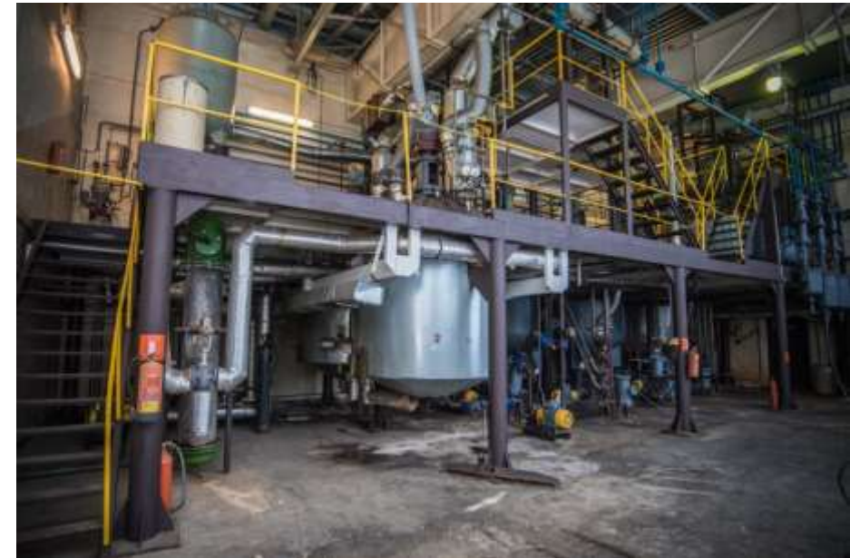
Polylabs production facility
